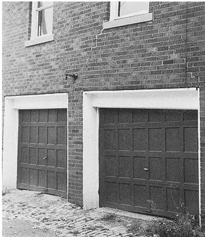
Figure 7. Subsidence damage. Tension cracks and differential settlement of walls and doors is typical (note door on right). (Photo by Ray Strawser)
